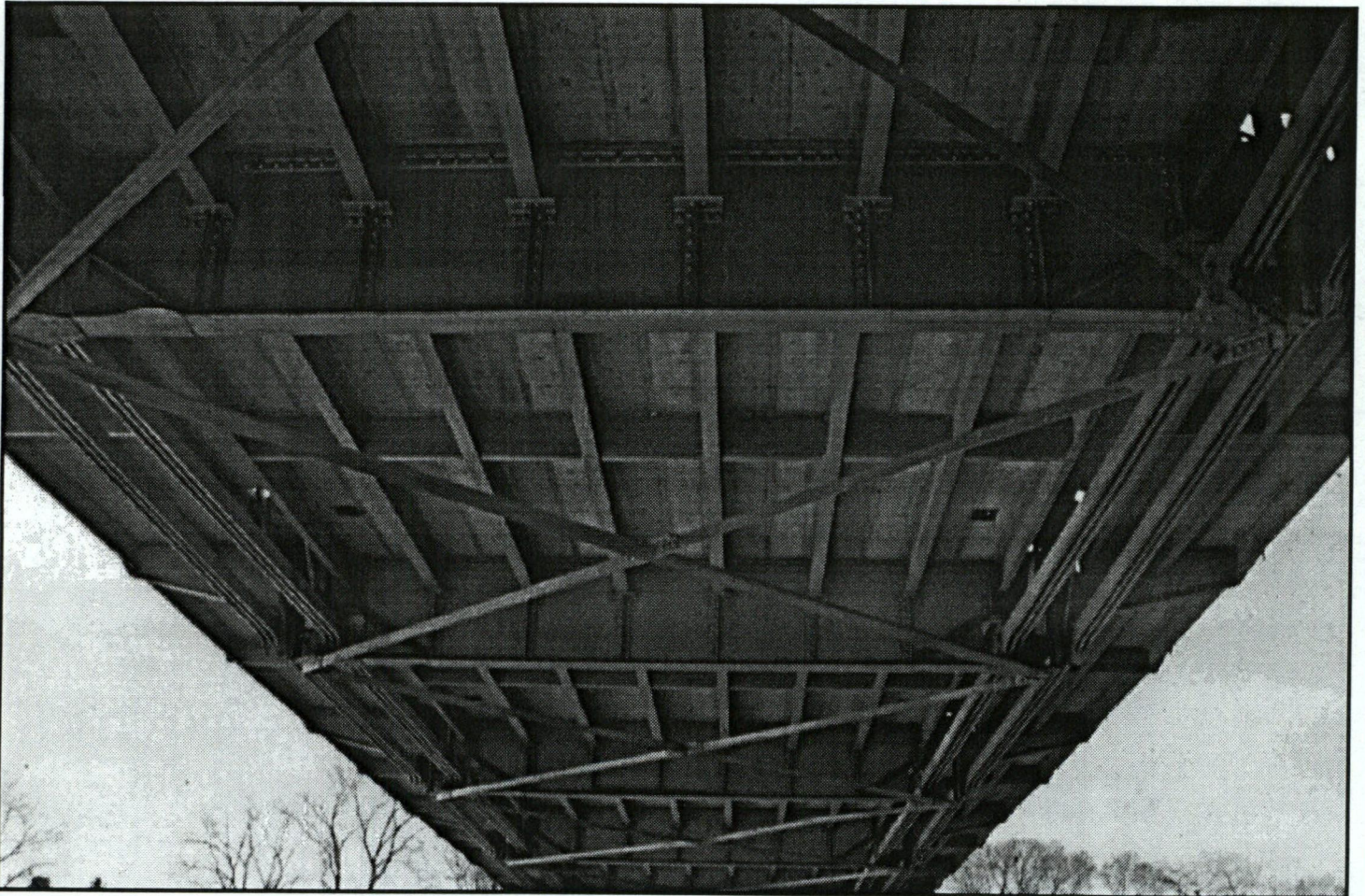
FIGURE 13 Decking supports Source: Author
