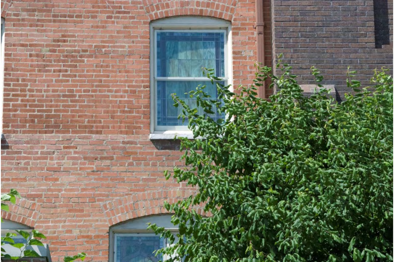
Photo 12: Rear (Northeast) Elevation, Detail, Brick Color Variation, camera facing southwest.
