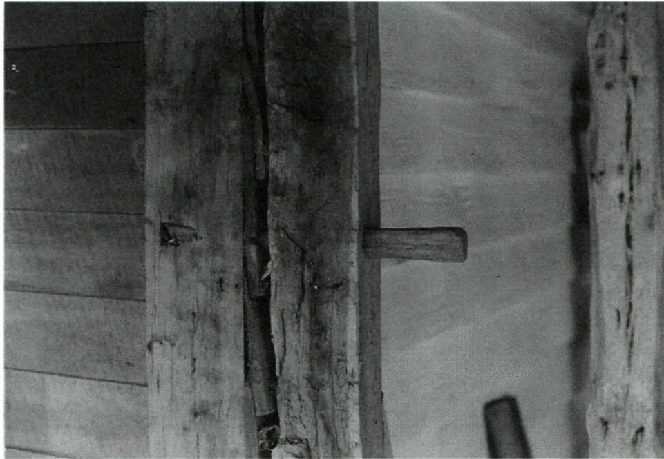
Figure 7: Photograph taken during 1986 restoration showing historic oak framing at breezeway with mortise and tenon construction. Courtesy Amy and Randy Walton.
