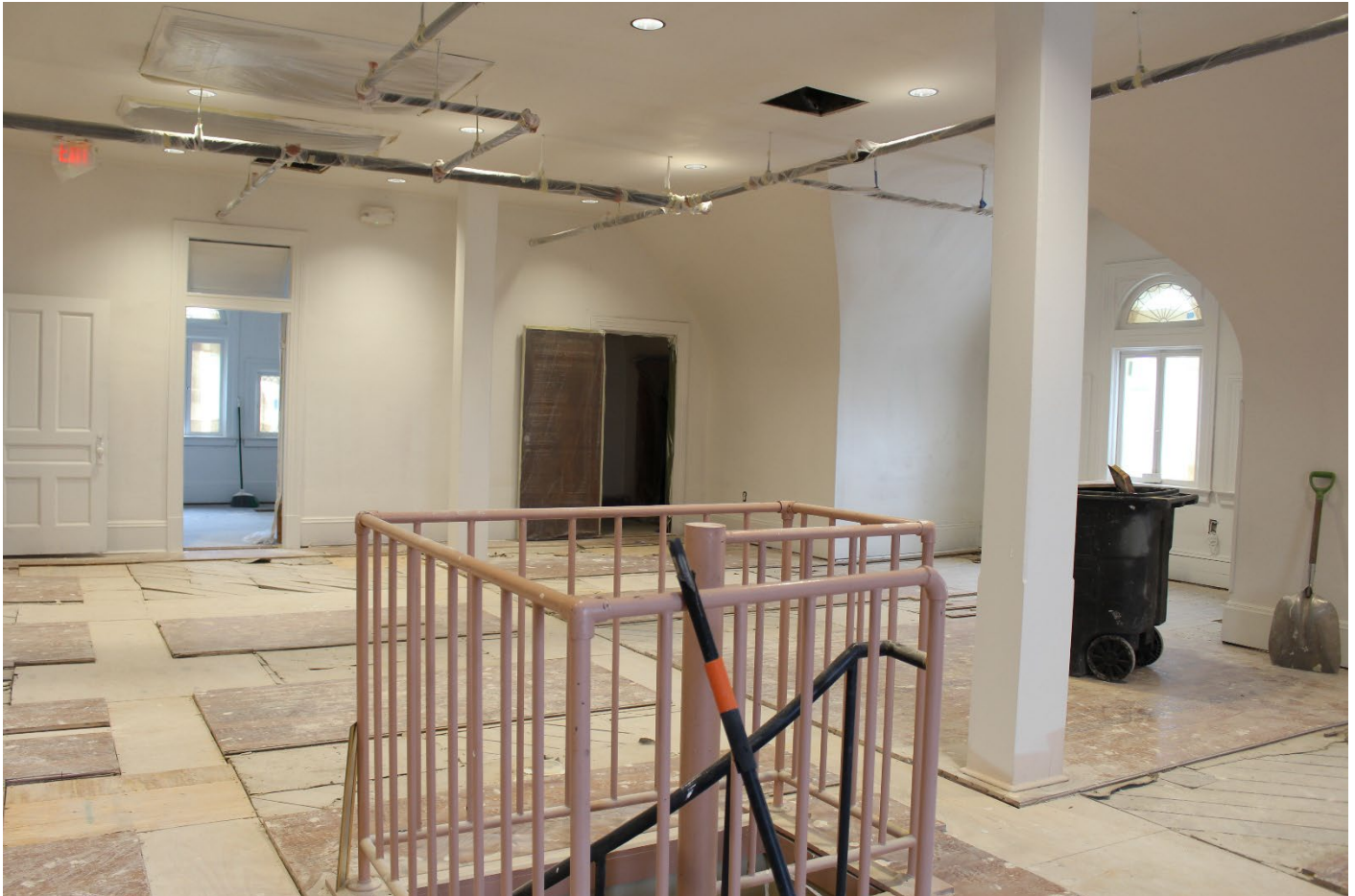
Photo 17. Koehler House – Third floor open interior space view to the metal spiral stair, camera facing northeast. January 30, 2026
