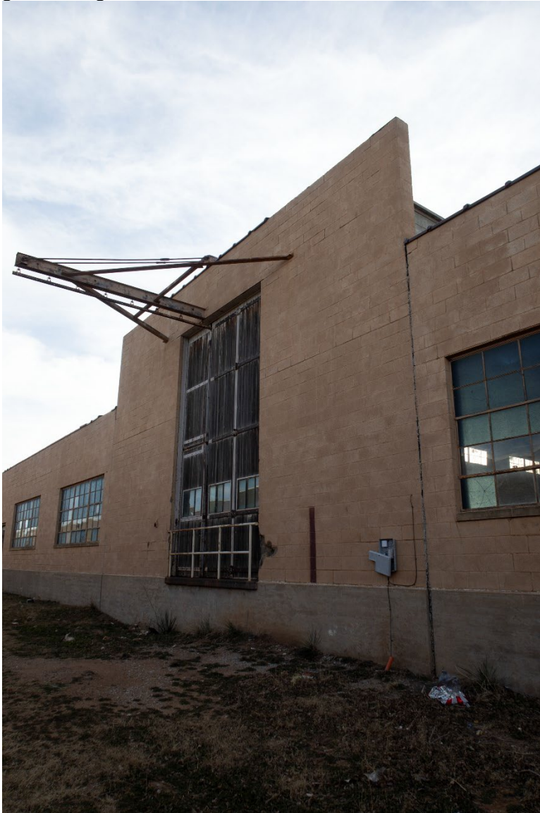
Photo 7. East elevation showing elevated roof monitor with original doors and equipment for loading and unloading glass, facing southwest.
