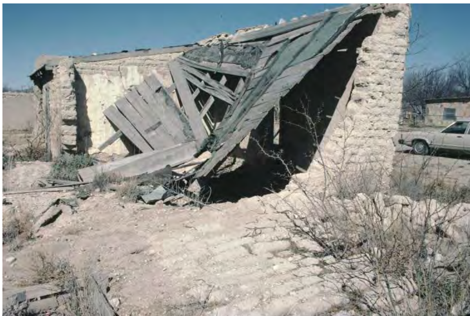
Figure 15. House with collapsed roof and walls, address unknown 1984 (Texas Historical Commission, Portal to Texas History)
