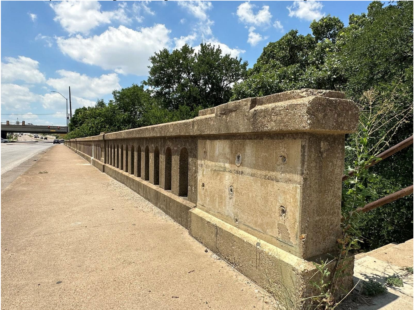
Photo 8. Oblique view of missing dado detailing on western column face. Camera facing northwest.
