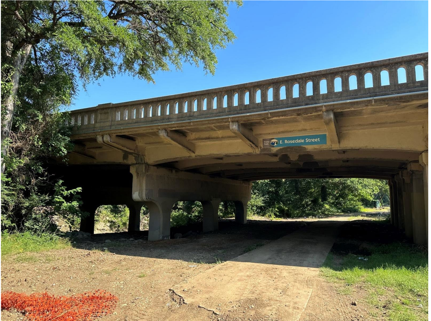
Photo 5. Oblique view of bridge substructure with street level railing, as seen from Sycamore Park. Camera facing northwest.
