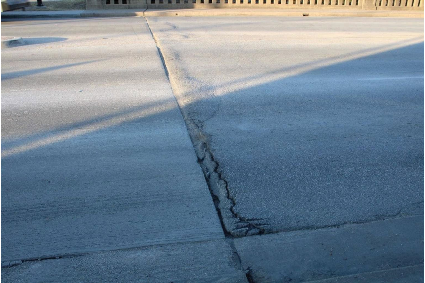
Figure 8. Detail of spalling at abutment joint. Source: William Schultz, Texas Department of Transportation Bridge Inspection Report completed February 9, 2022.
