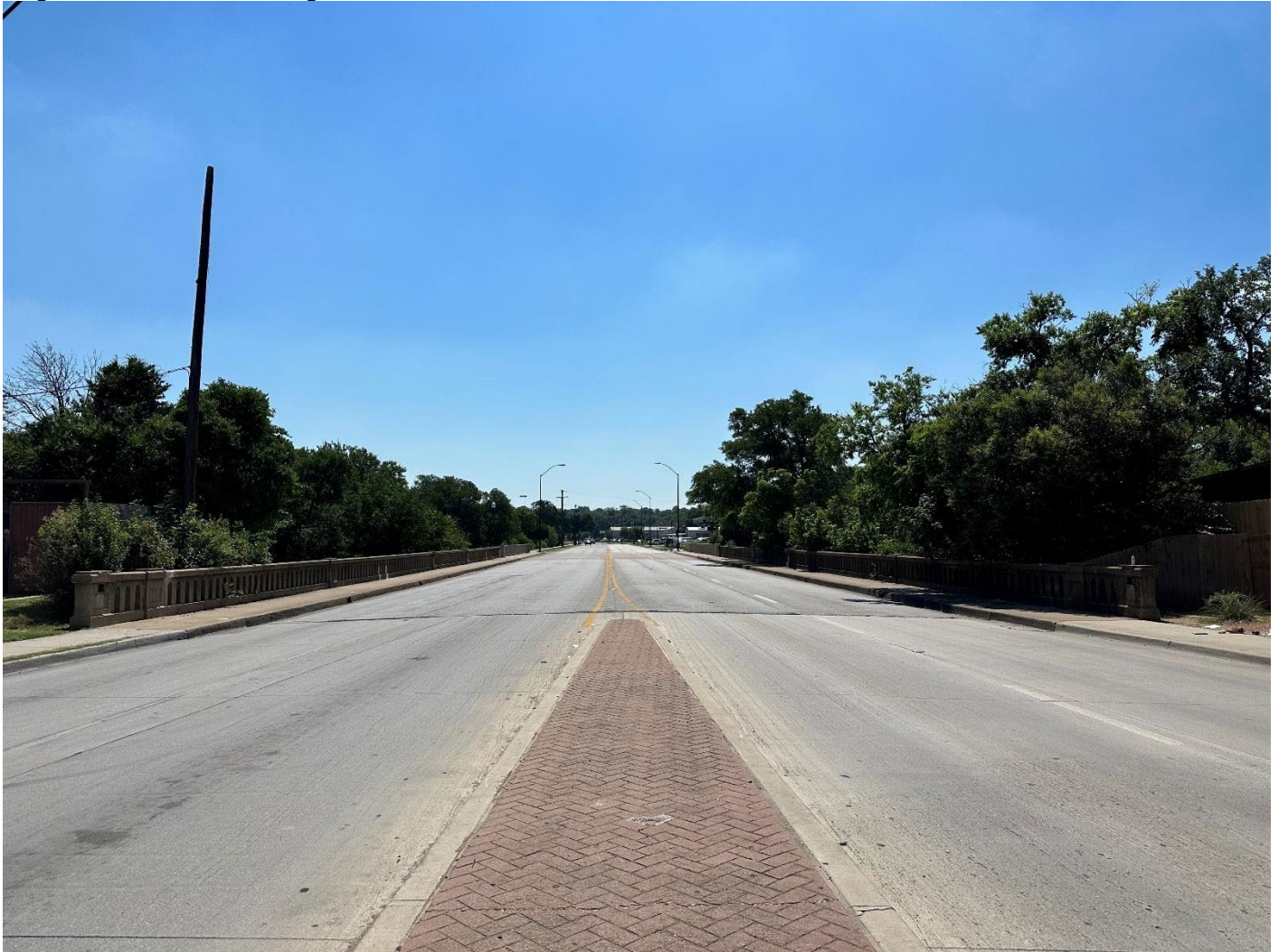
Photo 2. Centered contextual view of Sycamore Creek Bridge on East Rosedale Street towards Polytechnic Heights neighborhood. Camera facing east.
