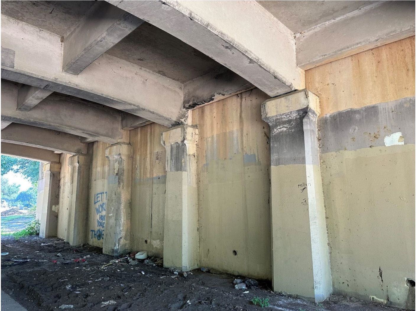
Photo 6. Oblique view the battered columns with decorative capitals that serve as the bridge seats for the girders of substructure. Camera facing northeast.
