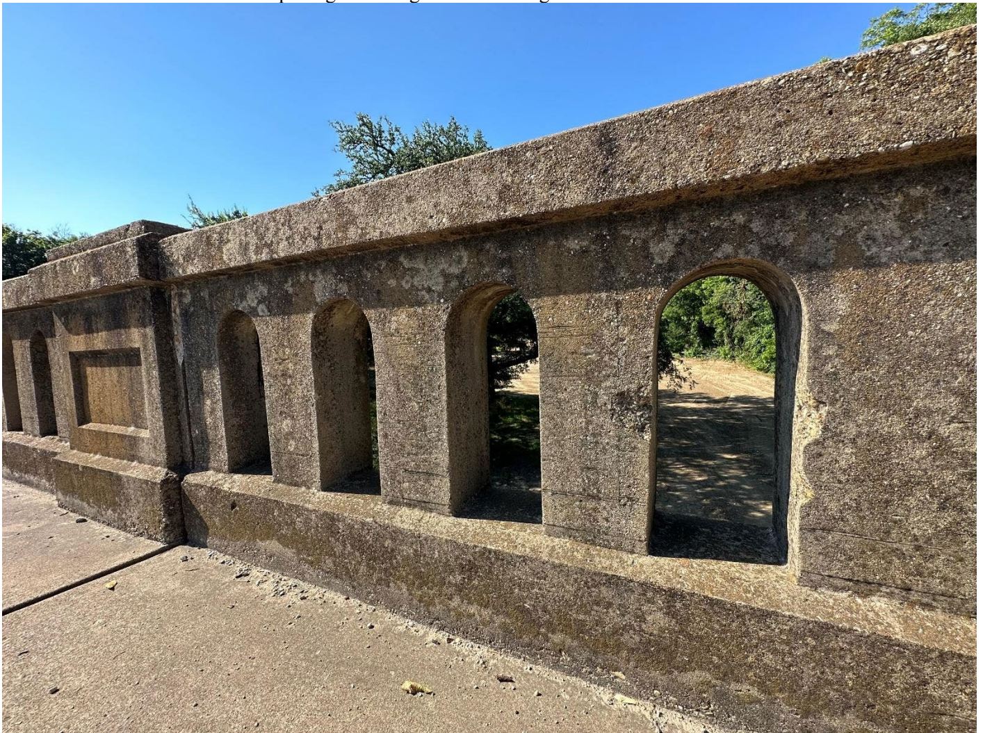
Photo 7. Detail view of concrete spalling on railing. Camera facing south.
