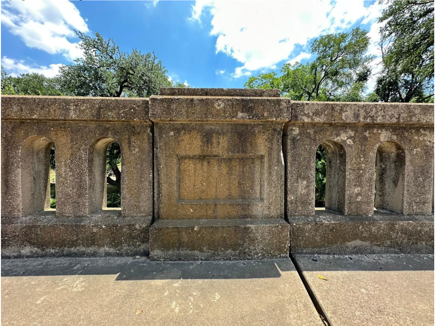
Photo 10. Detail view of railing featuring arched windows separated by a column with classical plinth, dado, and coping. Camera facing south.
