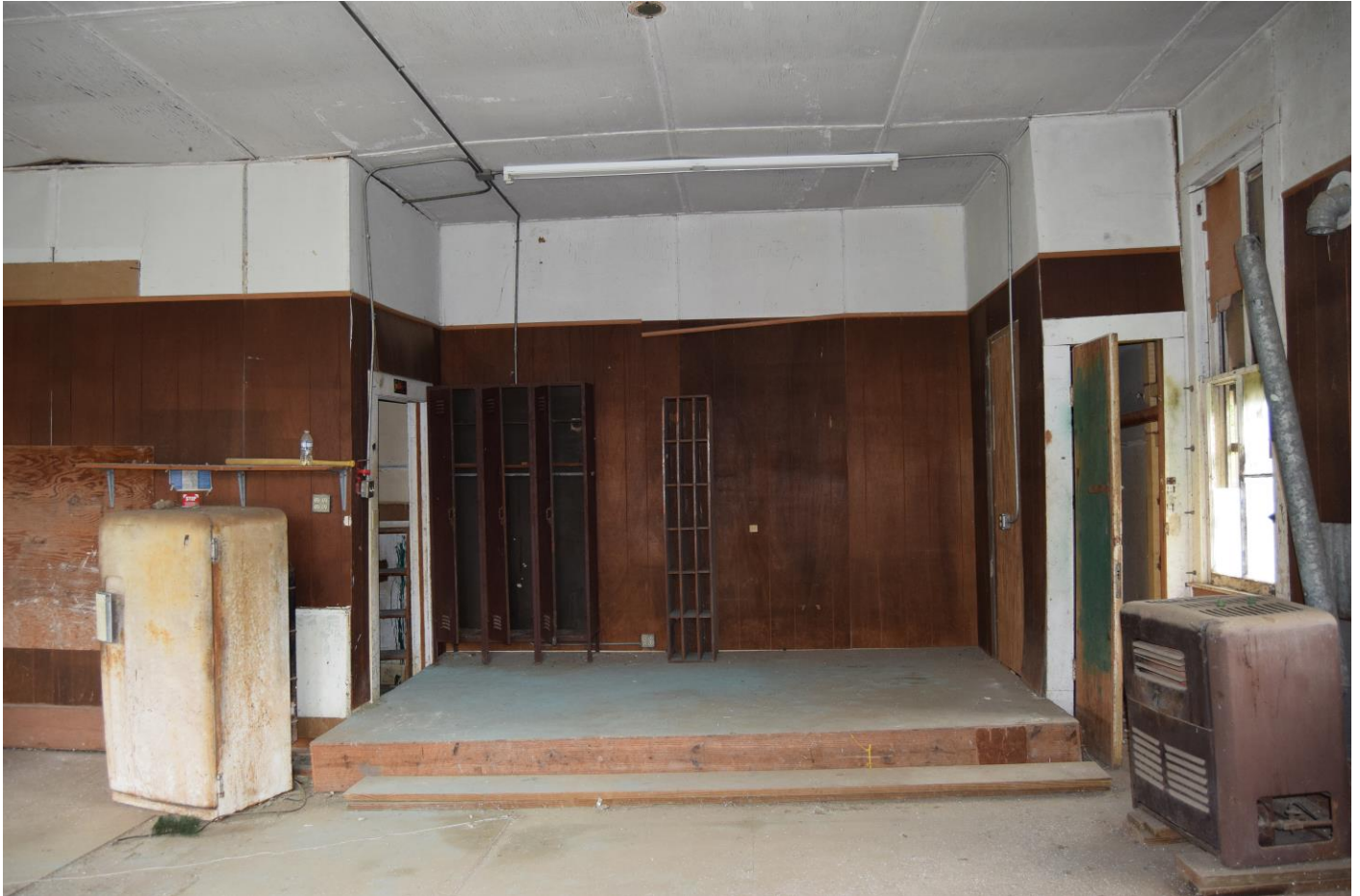
Photograph 9. Northwest wall of interior with platform at center and closets at ends, view facing northwest.
