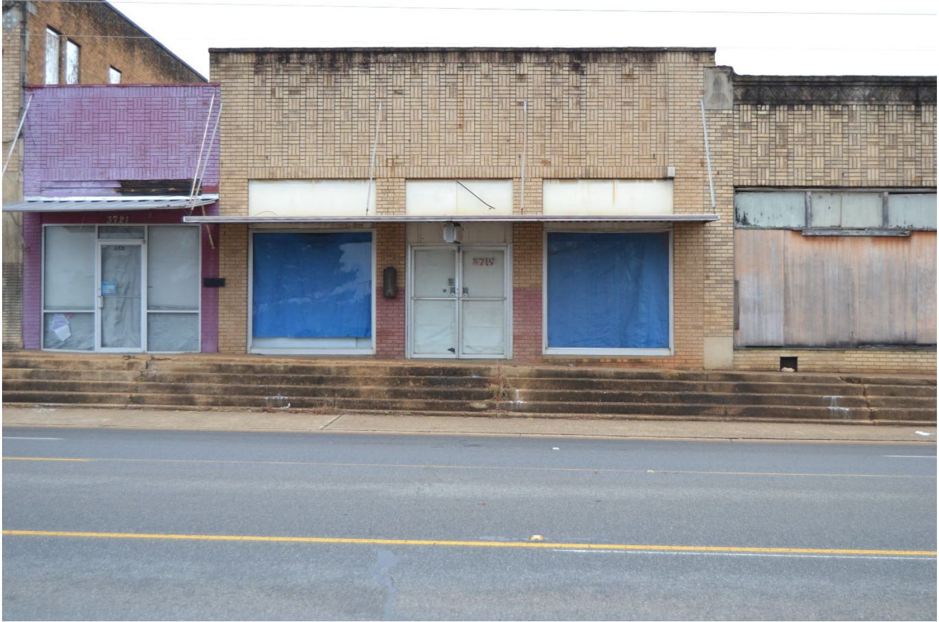
Photo 9. Camera facing north showing Resource 3 at 3719 West Marshall Avenue. Resources 2 and 4 are pictured to the left and right, respectively.
