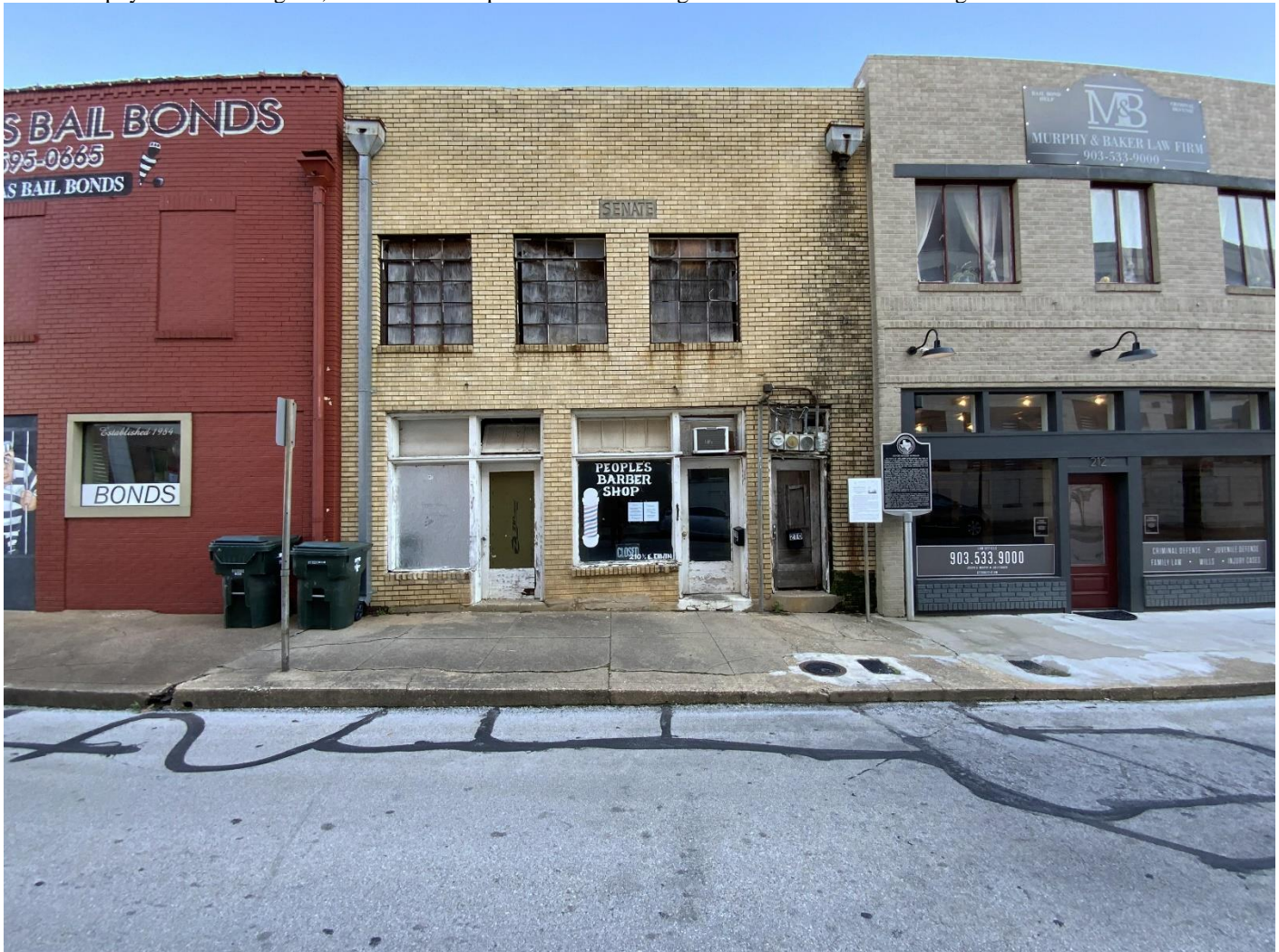
Photo No. 27. View of the Senate Building (Resource 58), located at 210 East Erwin Street. Archie S. Senate, an African American physician and surgeon, ran his medical practice here starting in the 1930s. Camera facing north.
