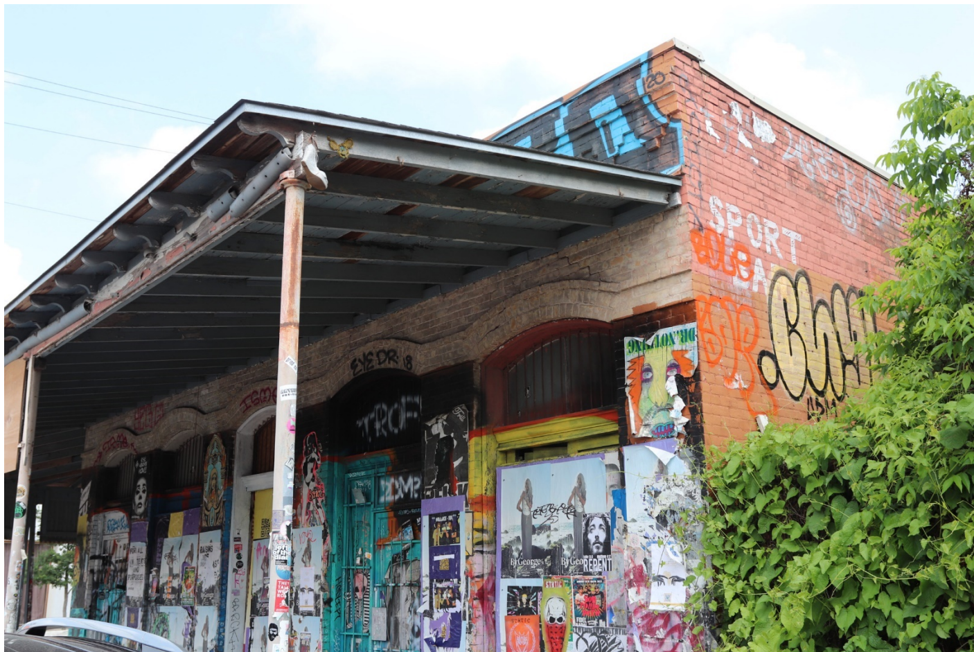
Photo 6: South façade detail showing decorative rafter tails and brick corbeling, facing northwest. Ghost signage for "Sport Bar" is seen on the east elevation, which is a solid brick wall.
