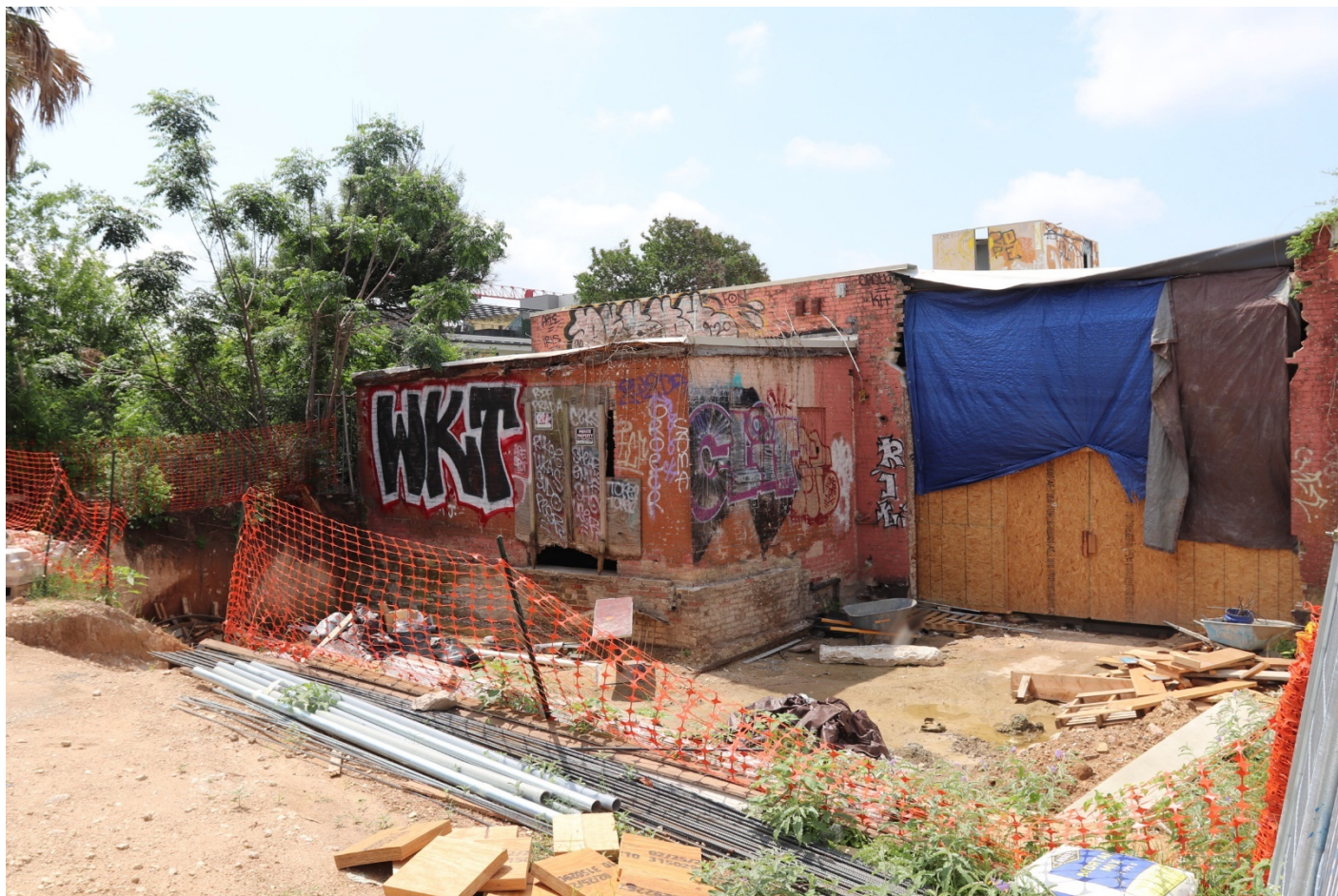
Photo 4: North (rear) elevation showing ongoing rehabilitation to the nominated building, facing south.
