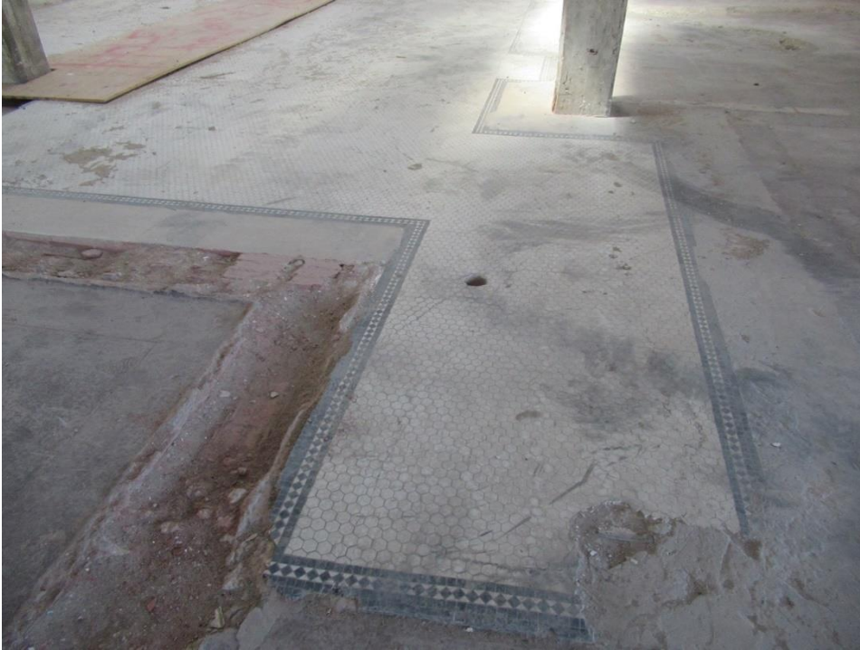
Photo 17: Second Floor Mosaic Tile Detail
