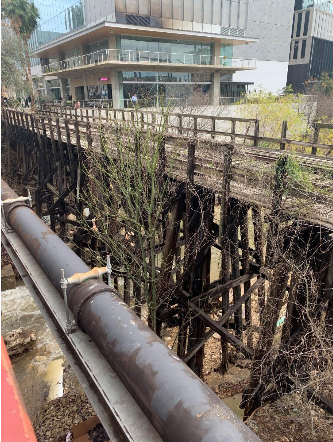
Photo 6: View of north side of Third Street Railroad Trestle, camera facing southeast. Photo by Andre Boudreaux.
