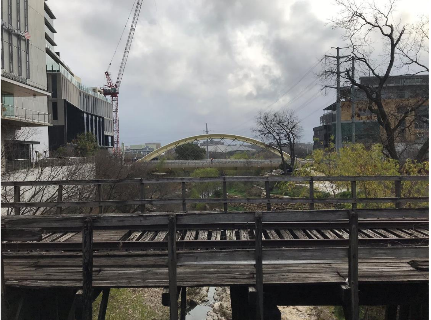
Photo 4: Third Street Railroad Trestle railing detail, camera facing south. Photo by Joemy Buschur.
