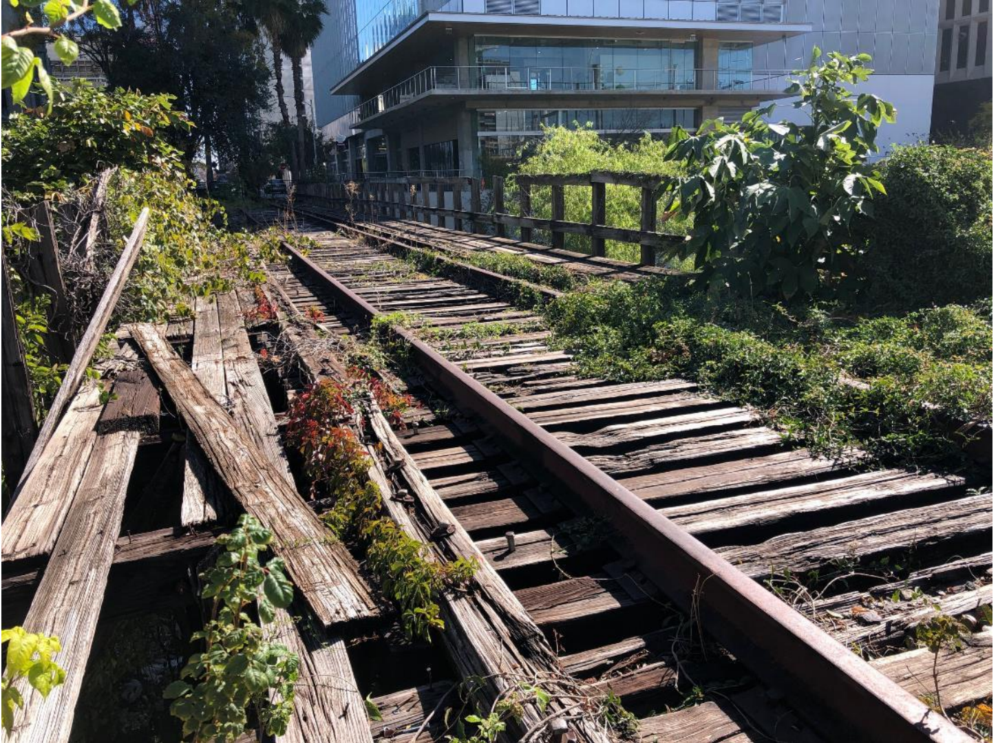
Photo 5: Third Street Railroad Trestle surface detail, camera facing east. Photo by Joemy Buschur.
