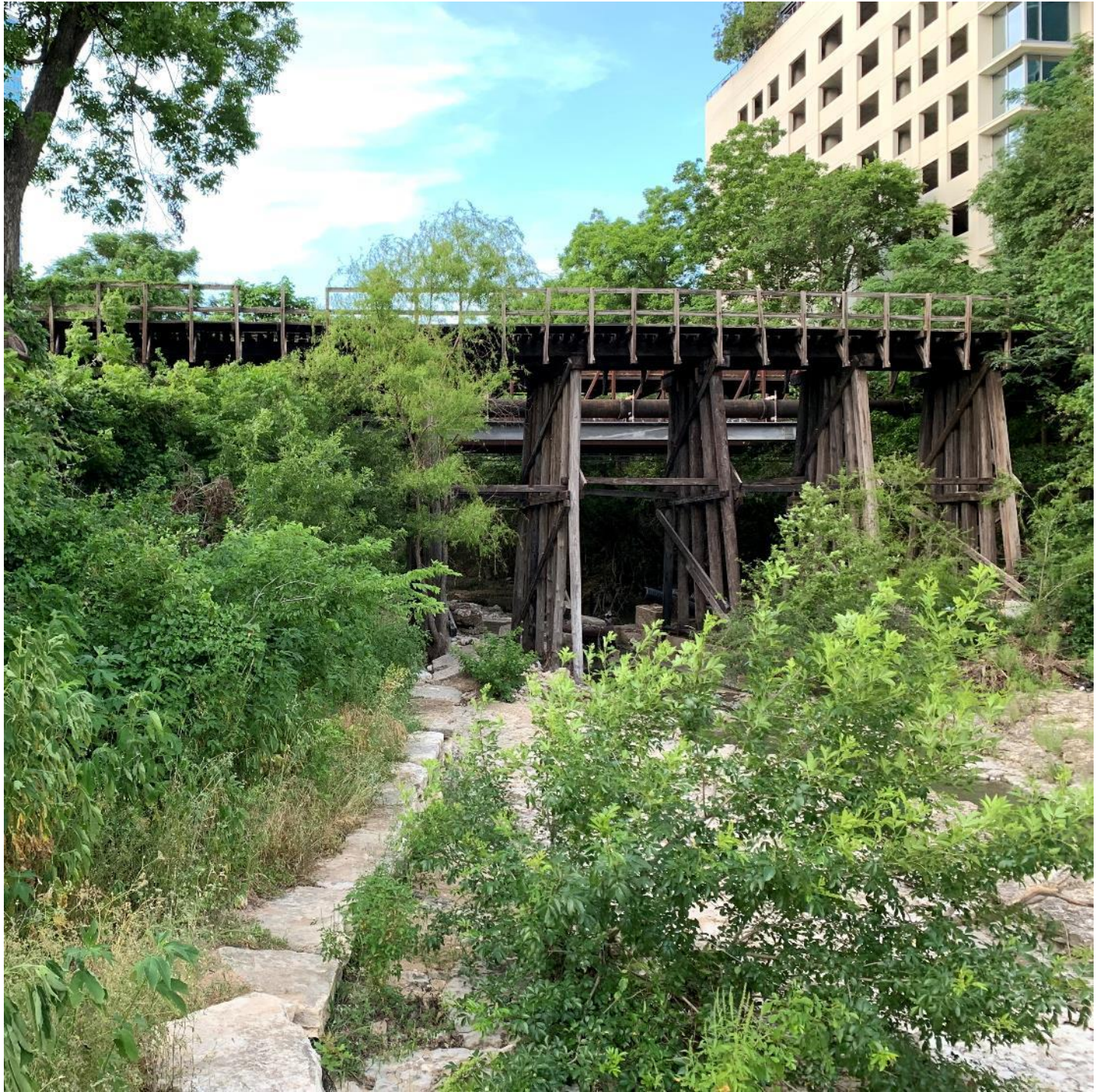
Photo 12: View of south side of Third Street Railroad Trestle, camera facing north. Photo by Andre Boudreaux.
