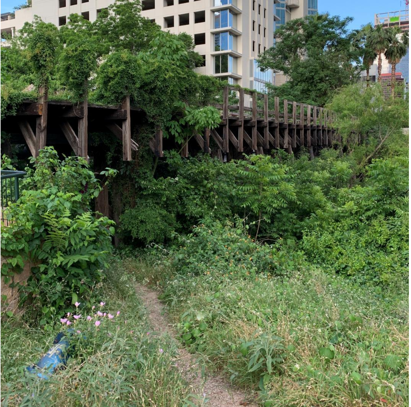
Photo 8: View of south side of Third Street Railroad Trestle, camera facing northeast. Photo by Andre Boudreaux.
