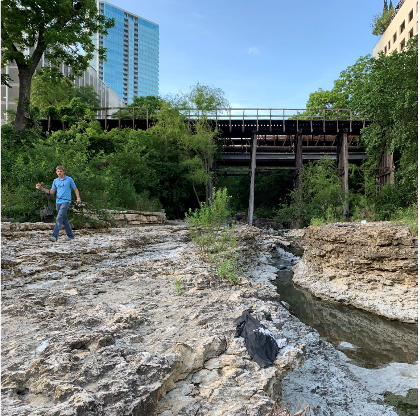
Photo 11: View of south side of Third Street Railroad Trestle, camera facing northwest. Photo by Andre Boudreaux.
