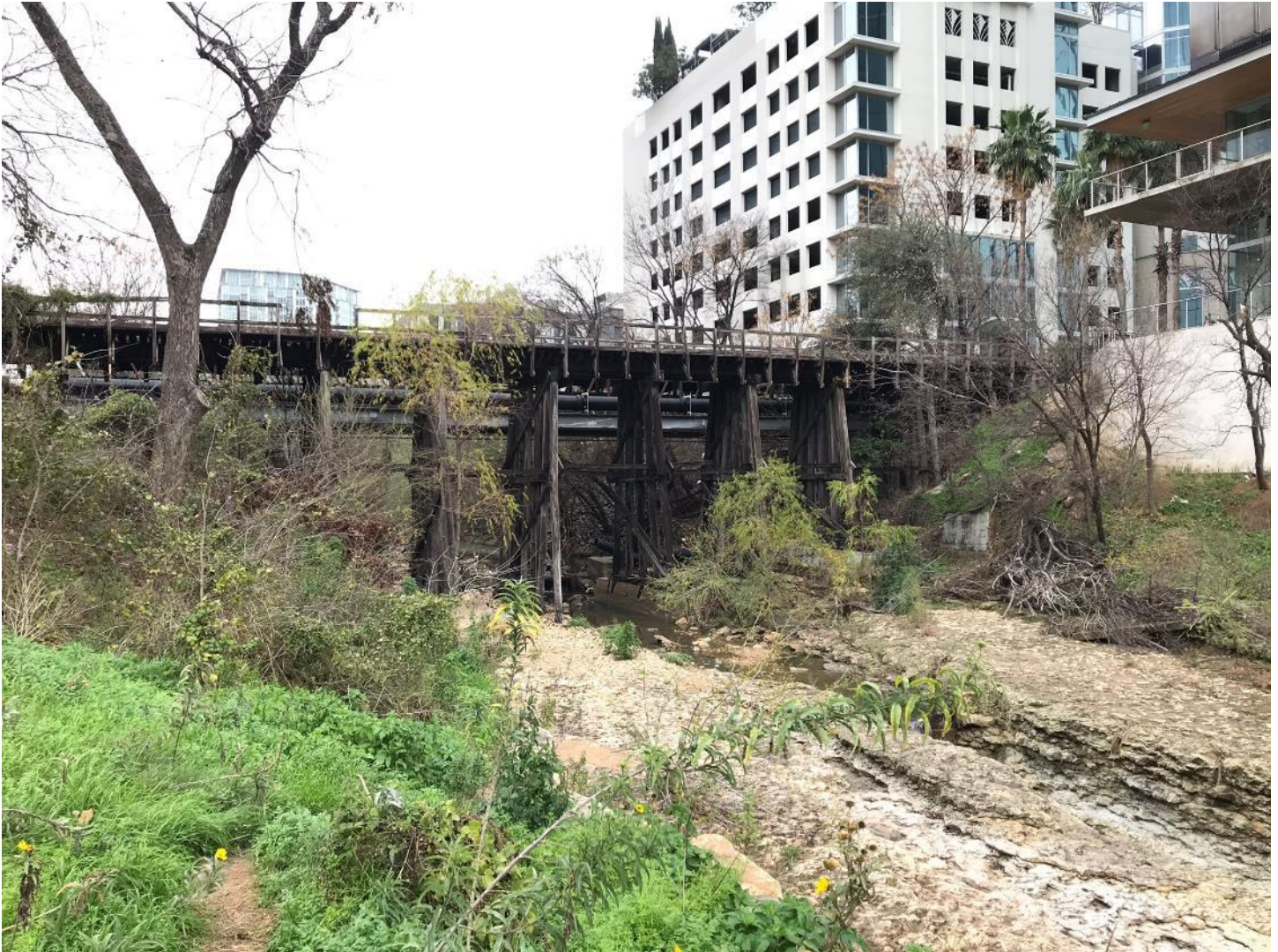
Photo 2: View of south side of Third Street Railroad Trestle, camera facing northeast. Photo by Joemy Buschur.
