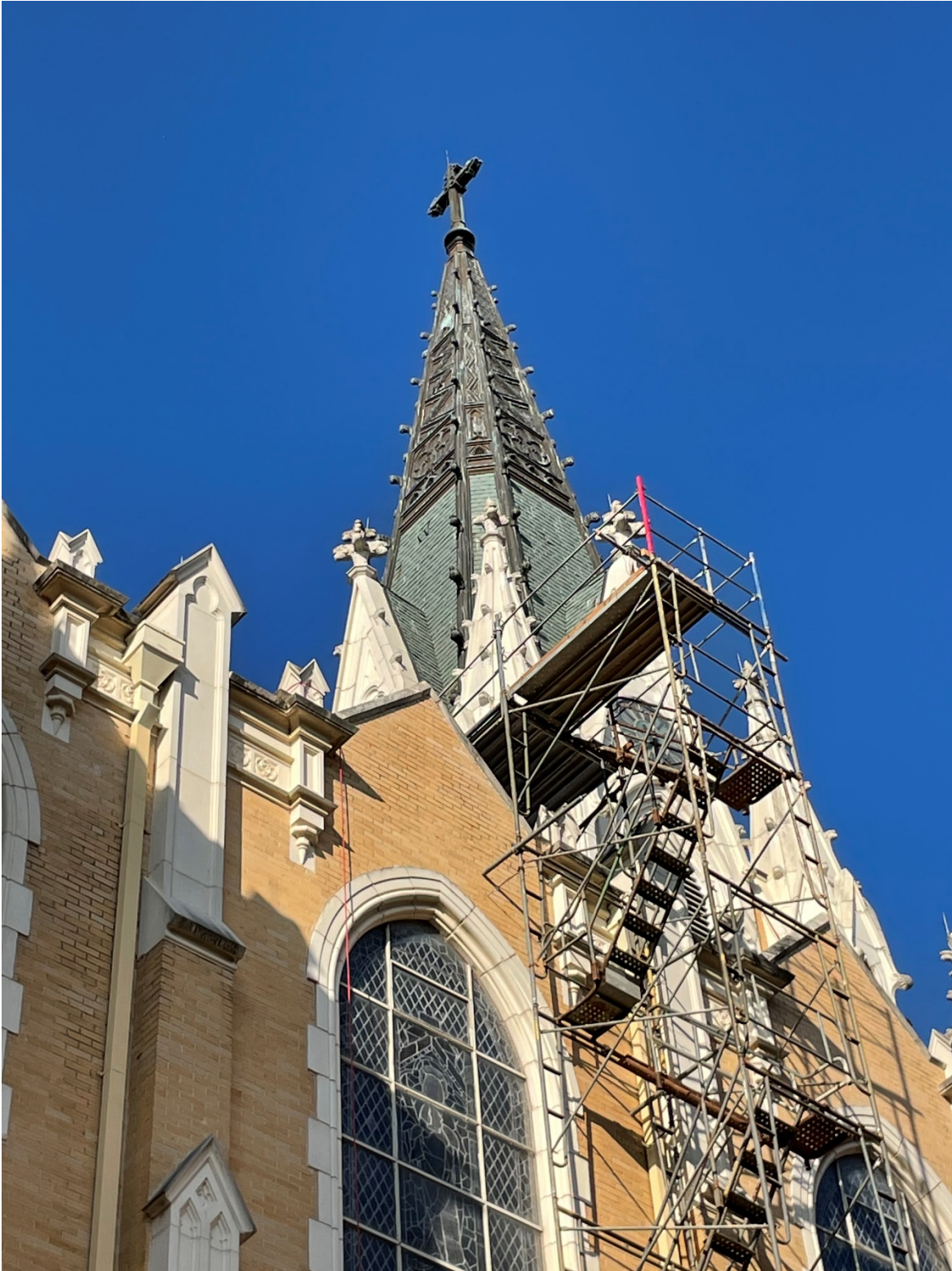
Photo 10: Tower spire with slate tiles, stamped panels, and cast stone cornice details. Looking northeast.
