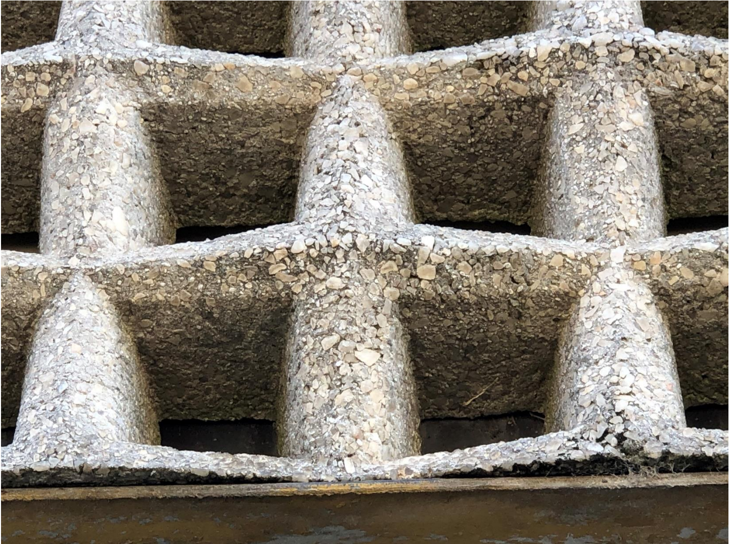
Photo 12 Brise soleil detail showing exposed aggregate September 2020
