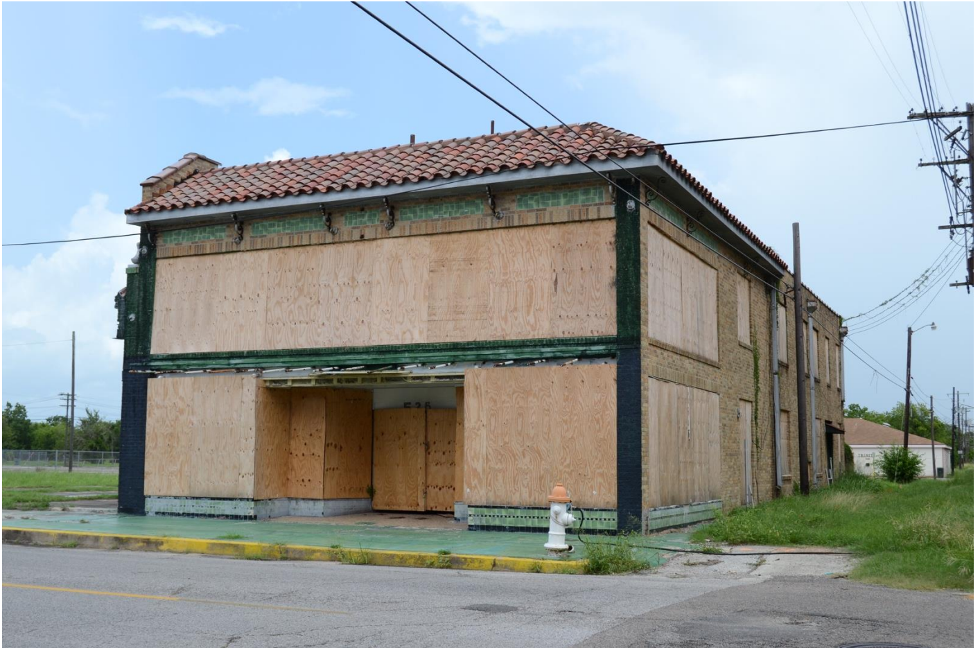
Photo 26. Oblique view of the Fred Miller Bicycle & Gun Repair/ Paint Shop building (Resource 4), facing north.
