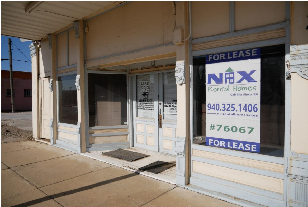
Photo 33. Mesker Brothers cast iron storefront at 212 SE 1st Avenue (Map ID 11725). Facing southwest.
