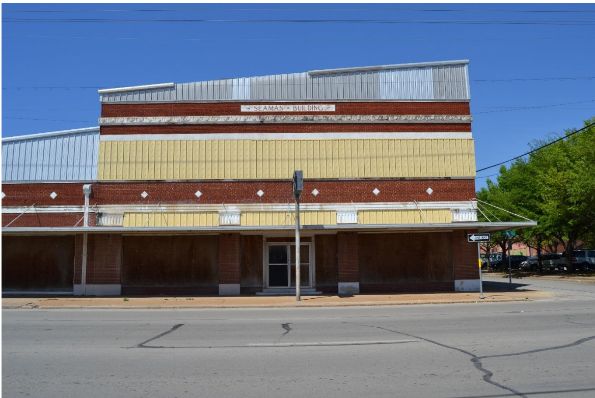
Photo 58. 200 W. Hubbard Street (Map ID 12399), an example of a historic-age noncontributing building.
