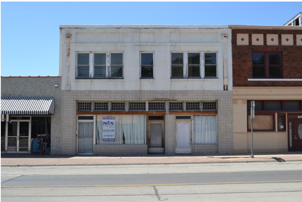
Photo 18. Façade of the Osborne Bath House and Hotel (Map ID 11835). Camera facing west.
