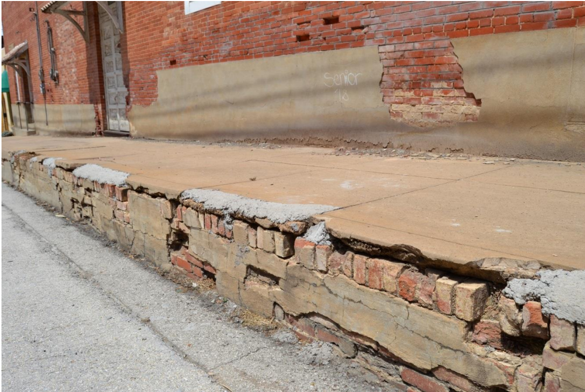
Photo 7. Original brick sidewalk found in the 100 block of NE 1st Street. Camera facing northwest.
