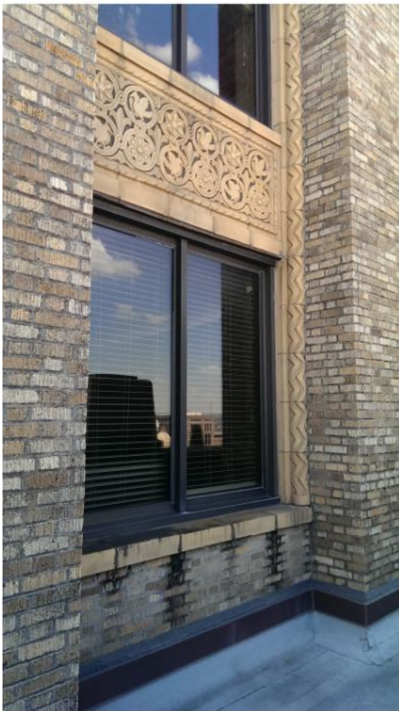
Photo 16: Exterior view of typical window at levels 17, 19, and 21 Camera facing north Date: 2015
