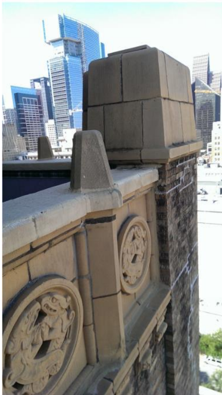
Photo 18: Exterior view of typical terra cotta detailing at parapet Camera facing north Date: 2015
