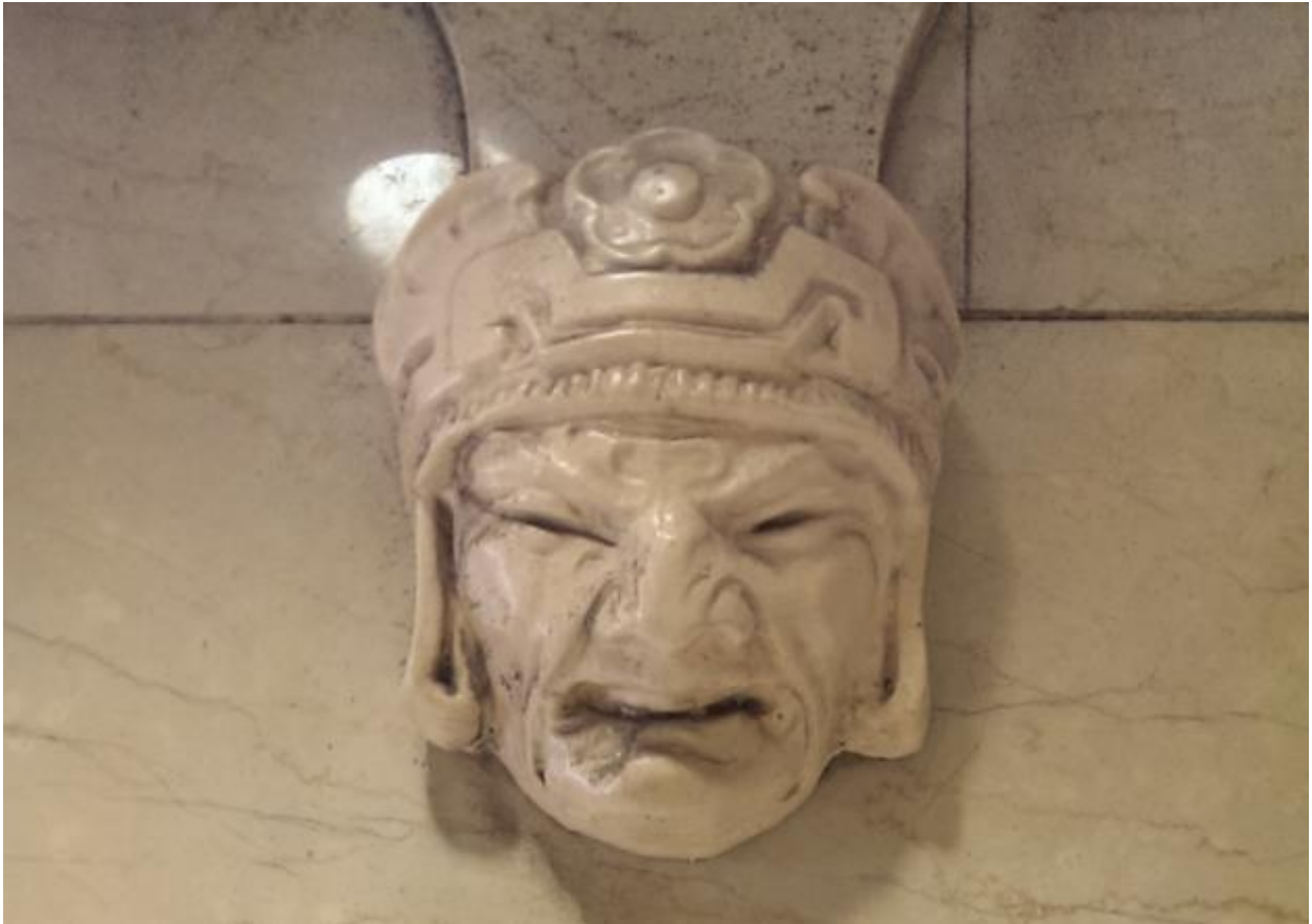
Photo 26: Enlarged view of Mayan stone detailing within ground floor elevator lobby Camera facing west Date: 2015
