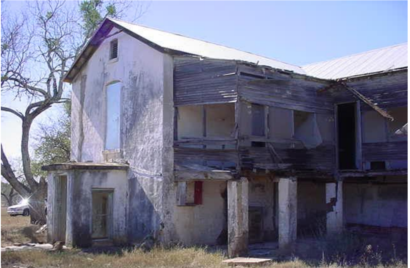
Figure 14: Resource A, Before Completed Work Source: San Antonio Conservation Society
