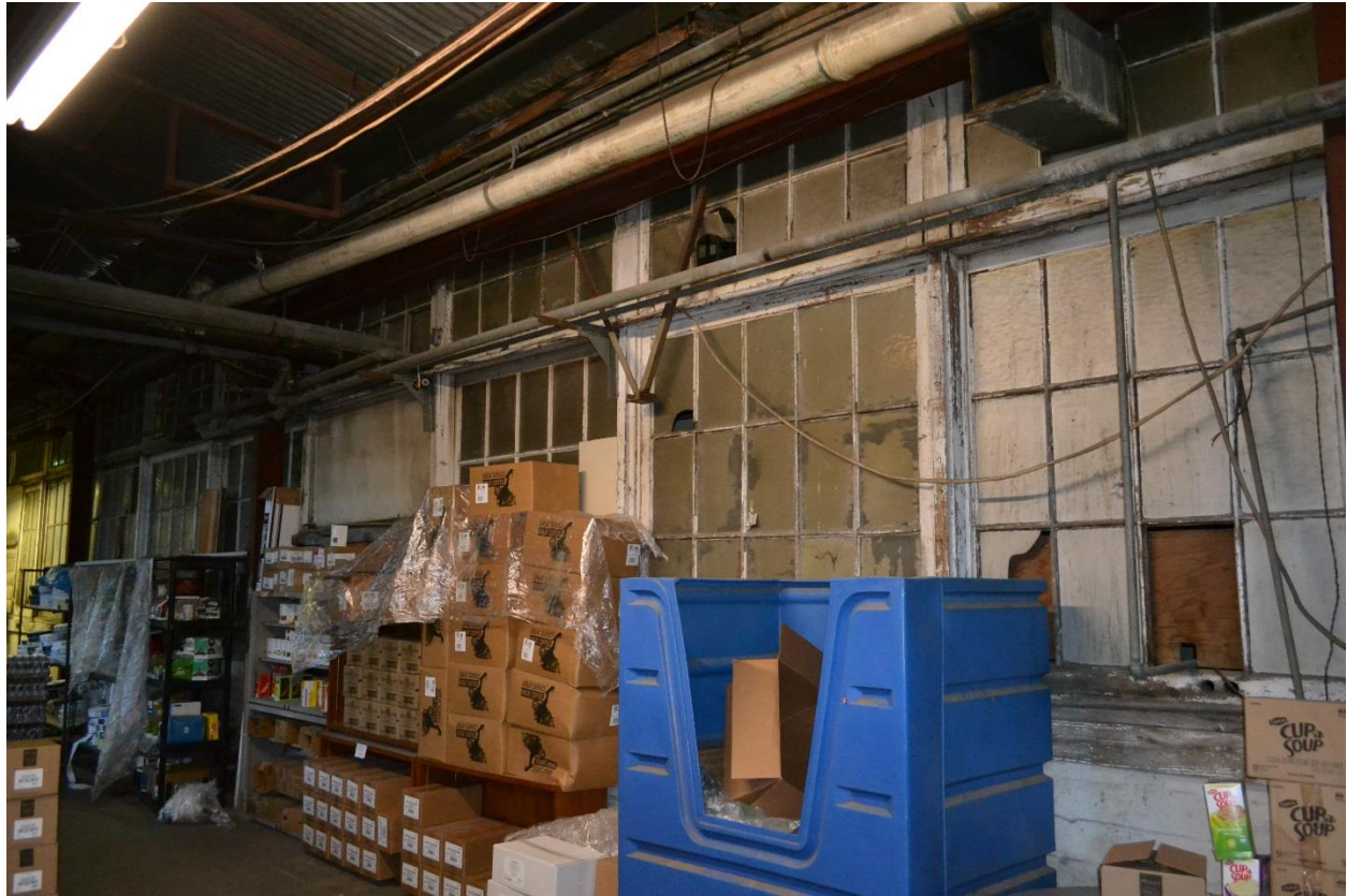
Photo 5 – East elevation of Building #2, #3, #4 with connection to Buildings #5 and #6, view southwest, October, 2017. The original metal windows and glazing remain in place.
