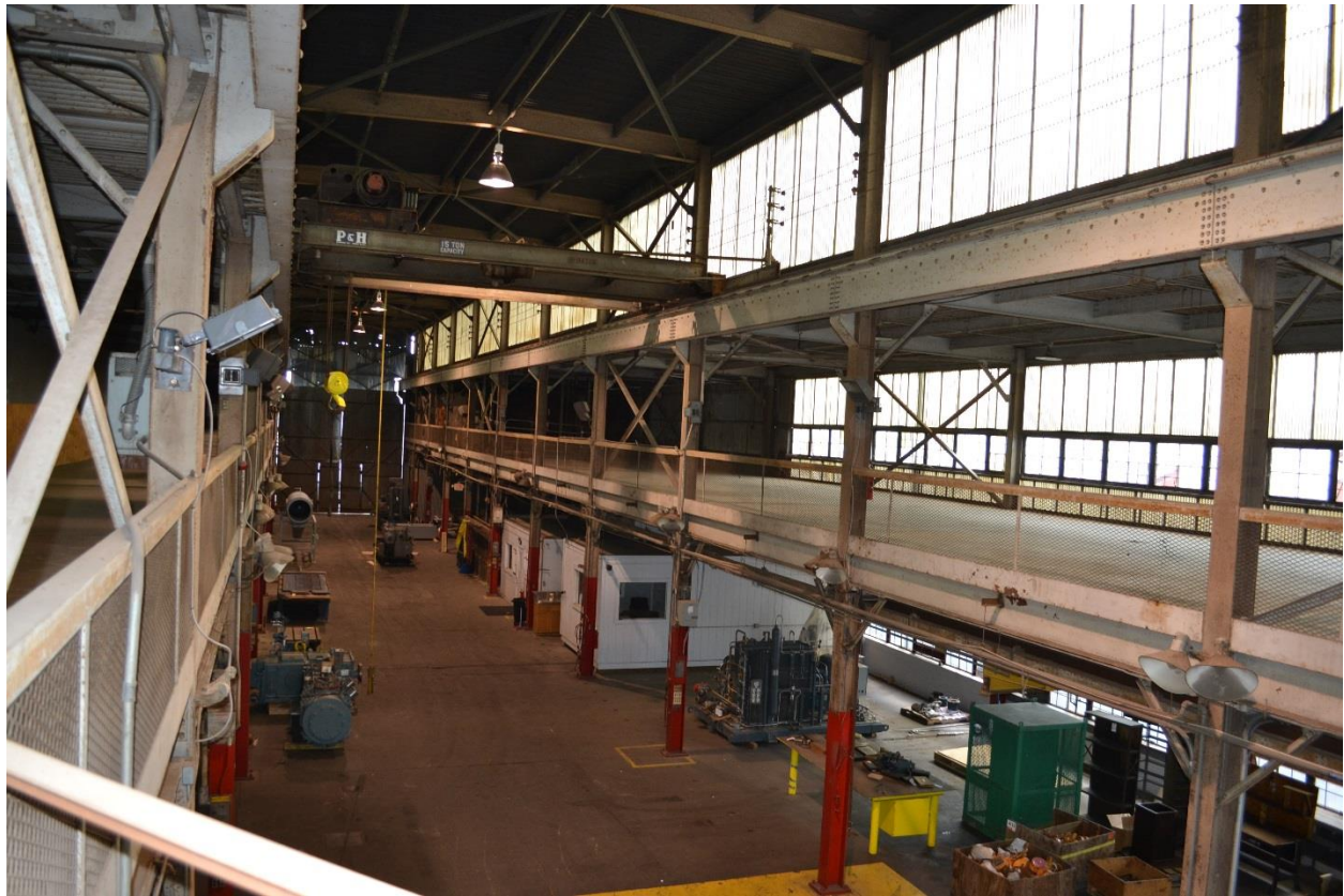
Photo 26 – Interior from second floor of Building #21, view northeast, June 2017. Original corrugated wire glass curtain wall, steel framing, and concrete flooring visible.
