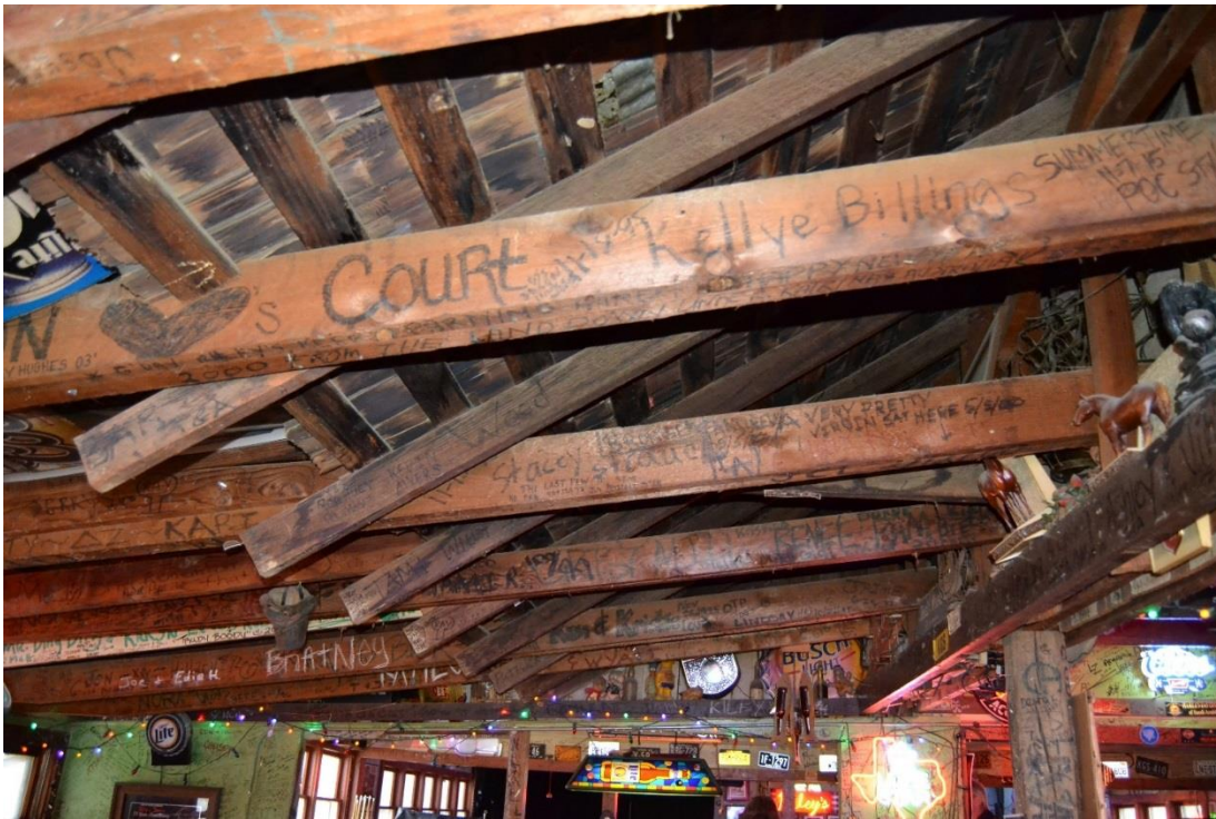
Photo 25. Detail of original roof truss system of Riley's Tavern (Resource #1), located in ca. 1935 addition of saloon.
