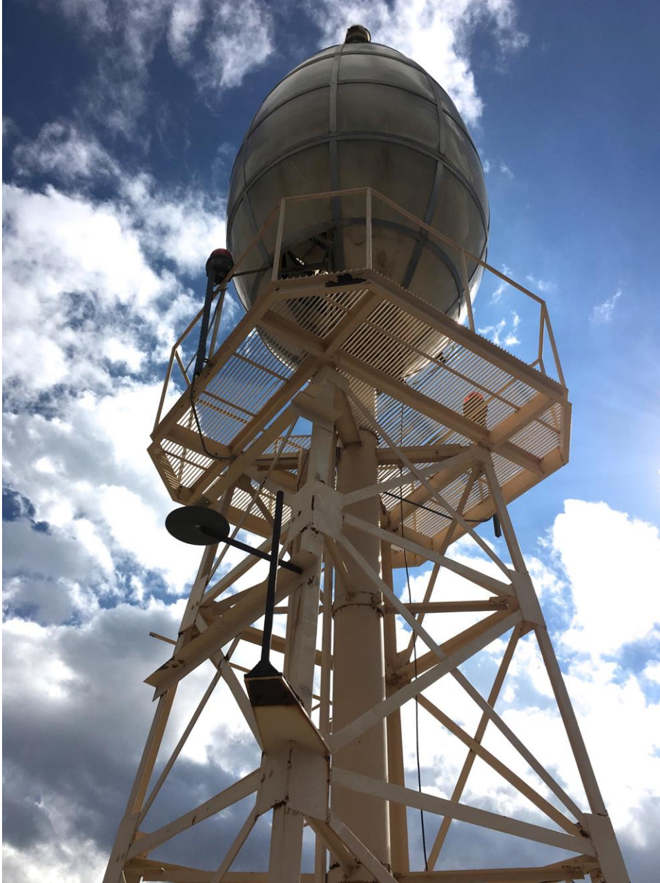
Photo 16 Flame Weather Beacon, looking up from roof
