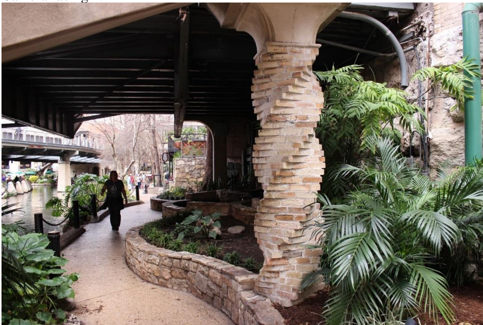
Photo 52 Block 15 (Crockett E Bridge S11 to Commerce Street Bridge / Jones Bridge S08) Twisted stair column Camera facing N
