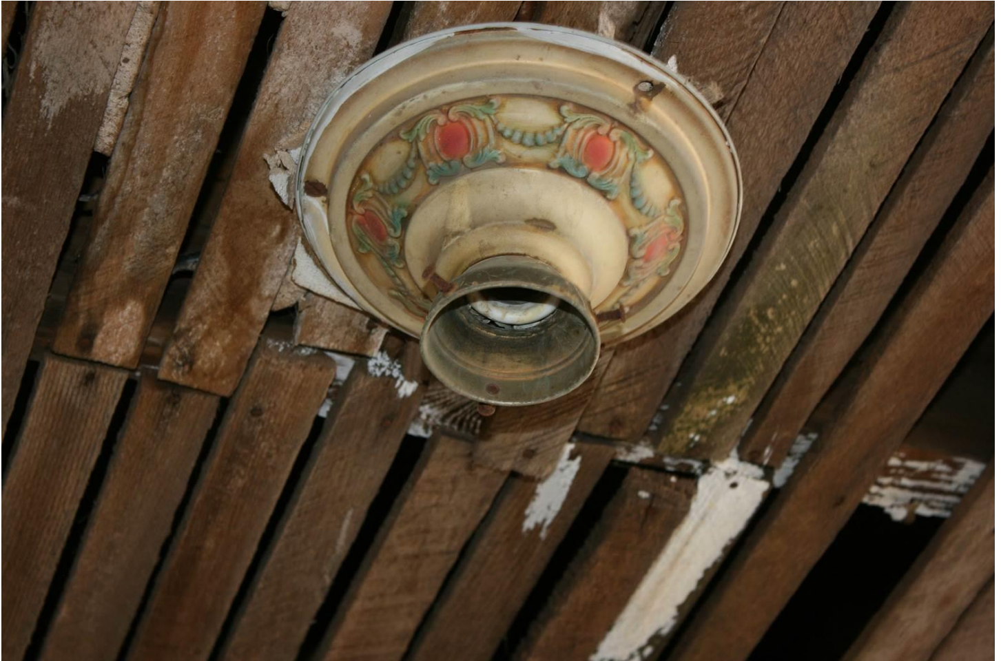
Photo 15: Second floor; decorated light fixture.
