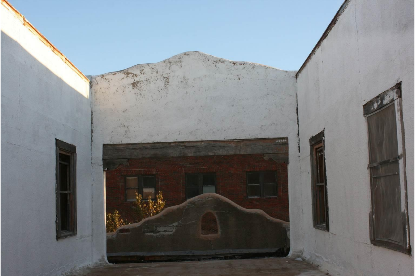
Photo 12: Second floor; West bay between two arms of E-plan. Camera facing south.
