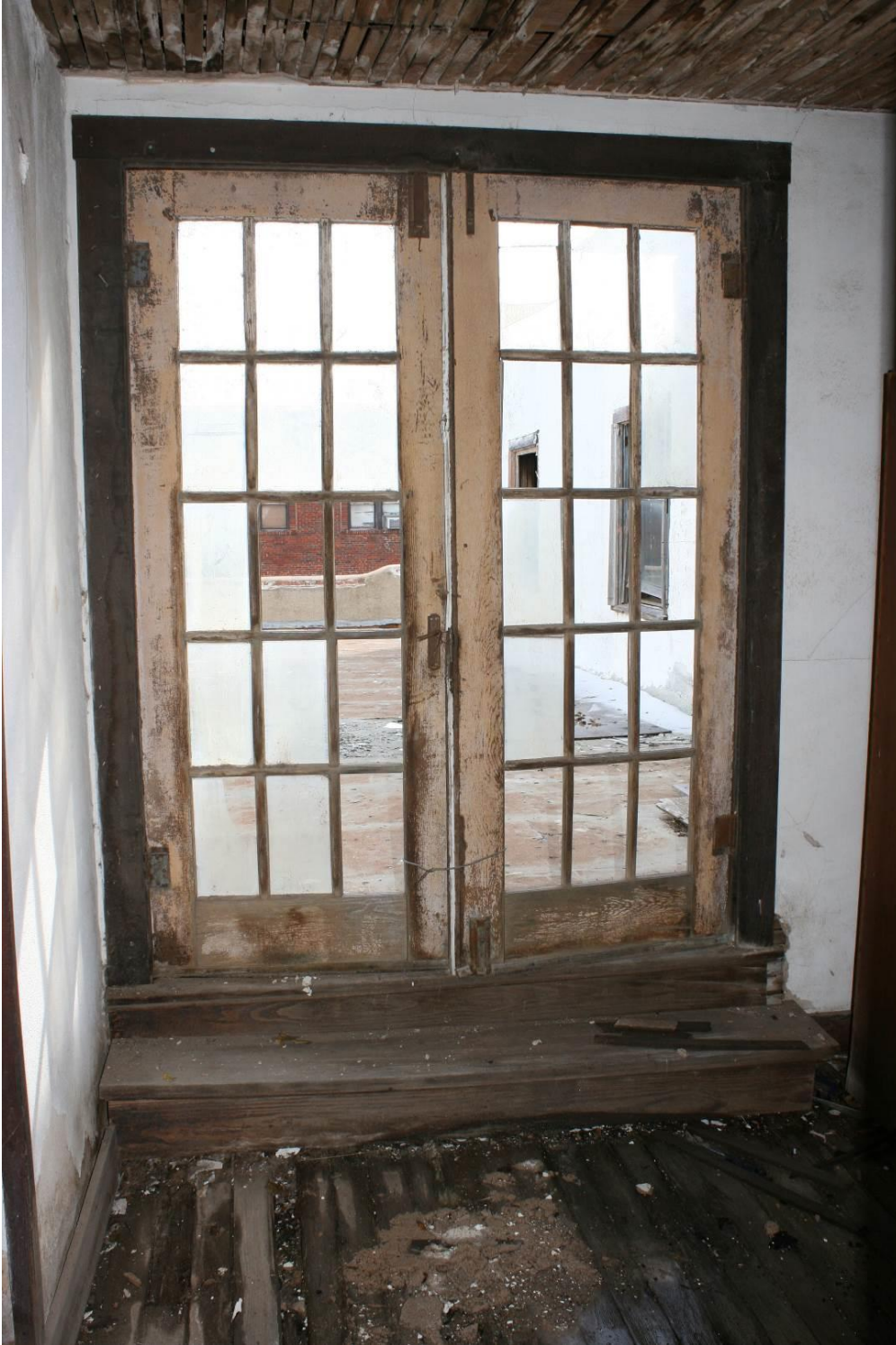
Photo 13: Second floor; double doors opening onto the east bay. Camera facing south.
